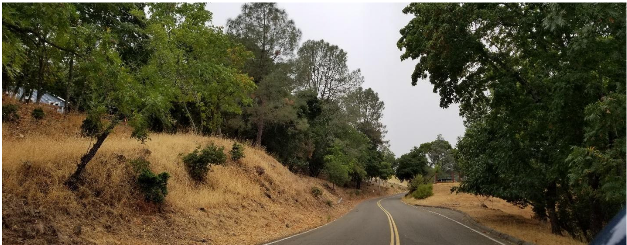
Photo 2. Example of maintenance needed along the road, where annual treatment of grasses and occasional ladder fuel (e.g. tree trimming and shrub removal) would be needed within 30 feet from roadside.
