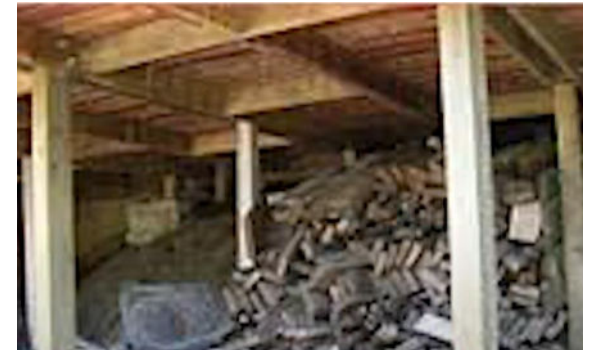
Nothing combustible under decks or stairs
