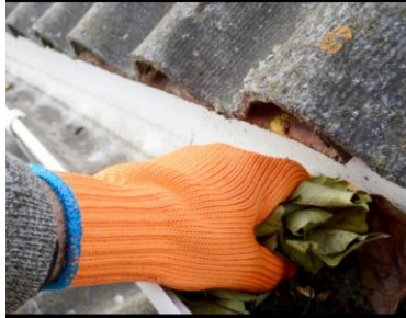
Debris from Gutter
