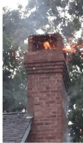
Keep branches 10' from Chimneys and Stovepipes
