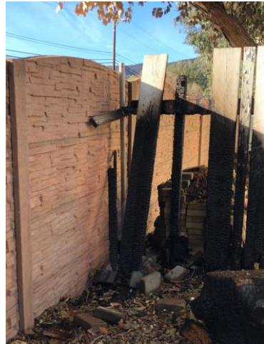
Fire-resistant gates and fence where attached to house
